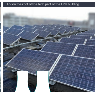
PV on the roof of the high part of the EPK building.
